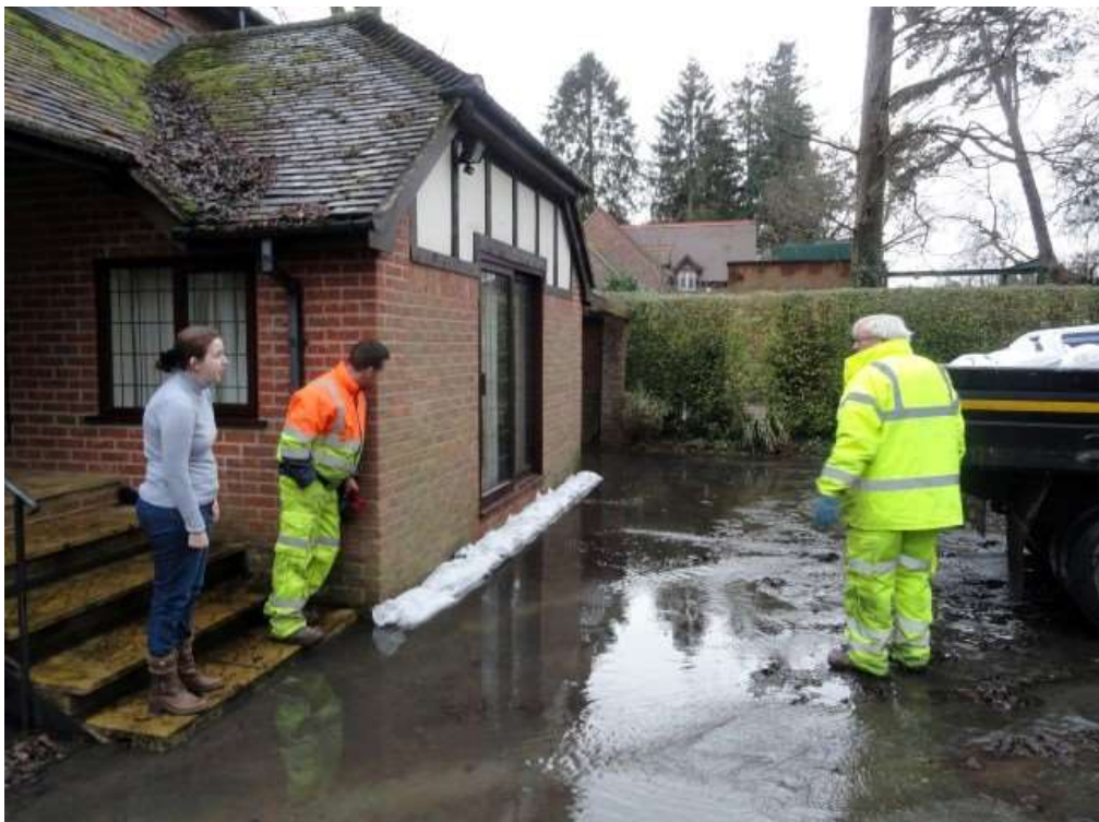
Figure 7 - Water from the restricted culvert flowing around the garden level room of Pavilion Cottage, Eastfield Lane
