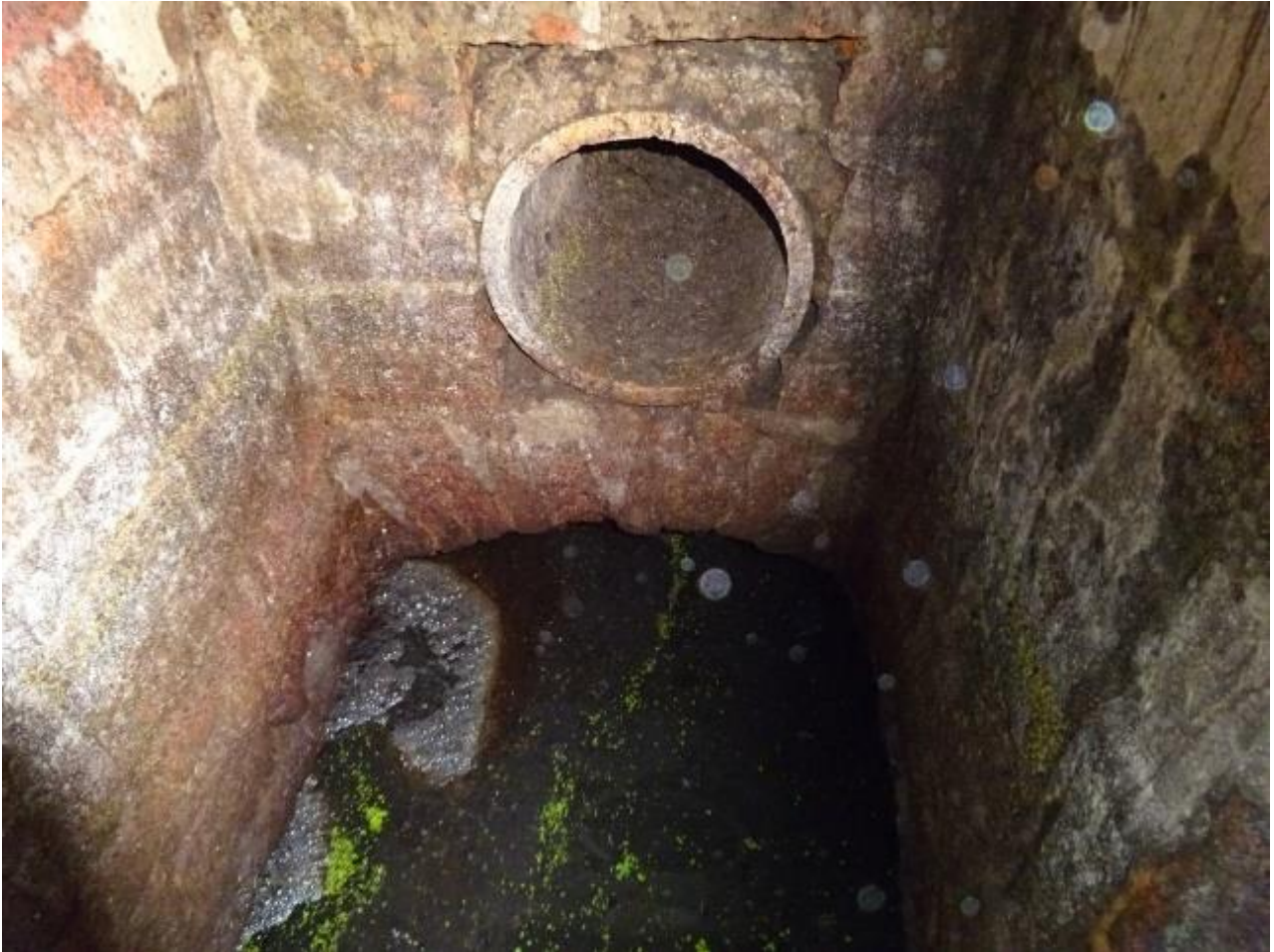
Figure 5 July 2020 photo of the chamber beneath the old fire station looking west, showing the arch of the culvert that crosses the High Street. Note the duck weed from the pond the other side of the road.
