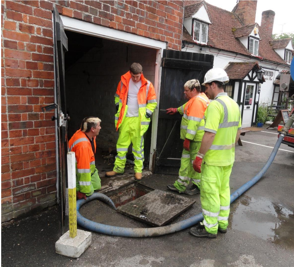
Figure 4 – the large chamber in front of and beneath the old fire station
