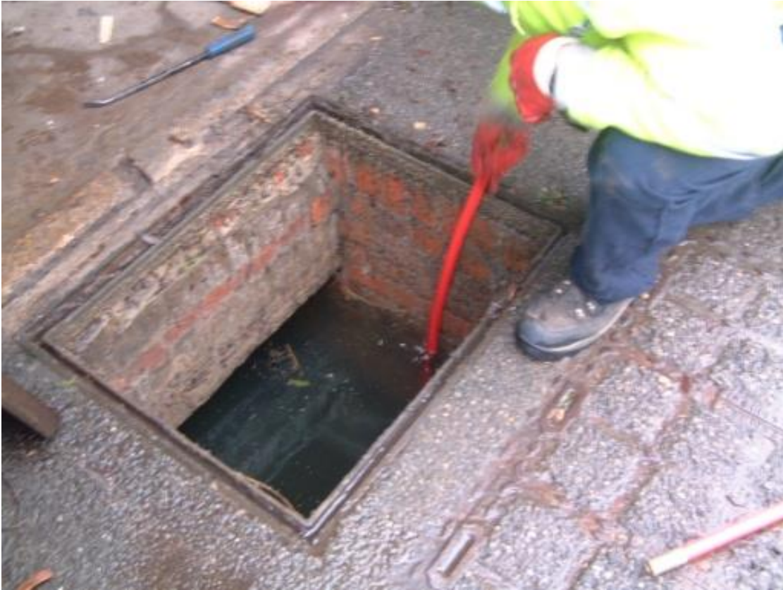
Figure 6 The 2 metre drain rod at the chamber's base. Compare the high water level in 2014 (ground water table to that of 2020 in fig 5)
